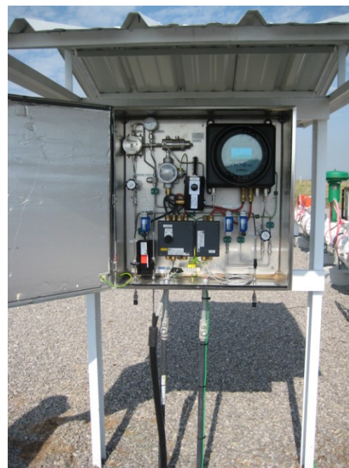
Condumax II Installed in outside Analyser house
