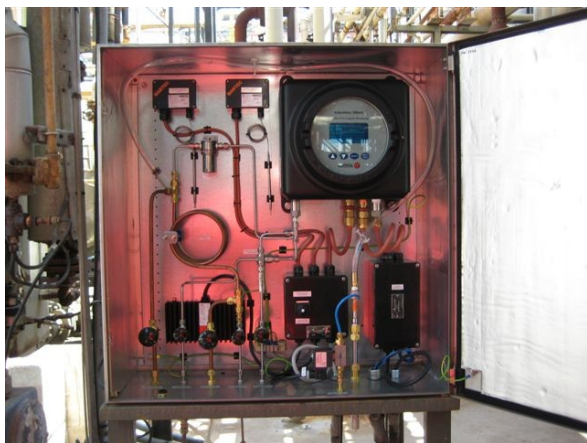
Liquidew EExd sampling system installed in process
