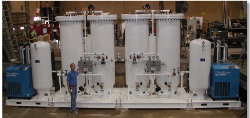
Fig.5 Skid mounted Pressure Swing Adsorber (PSA)
