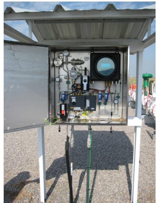
Condumax II Installed in outside Analyser house
