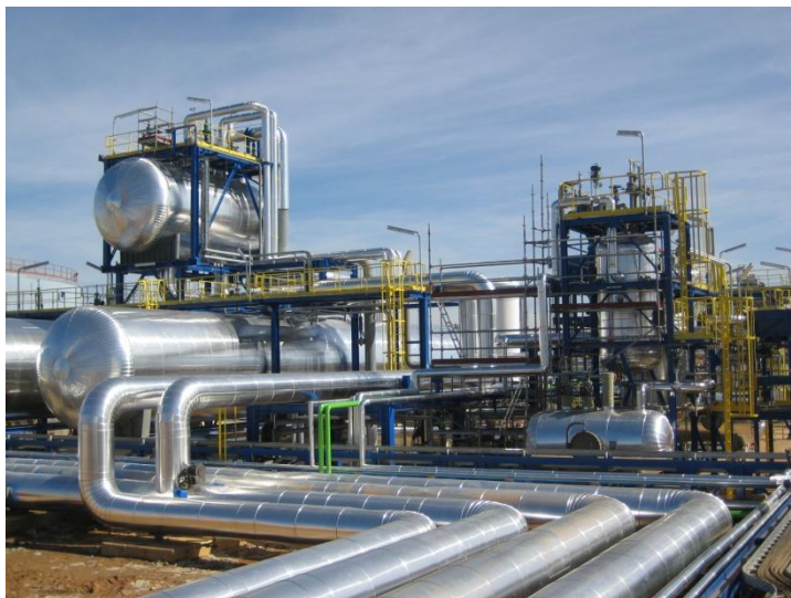
Moisture separation tank and condensers
